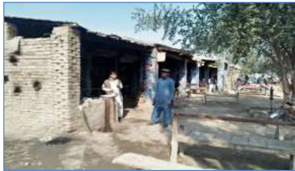
Plate 48: A view of Affected Structures at Zoorgrah
