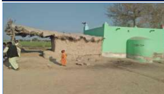
Plate 33: A view of affected mosque and thatched shed at 138+950
