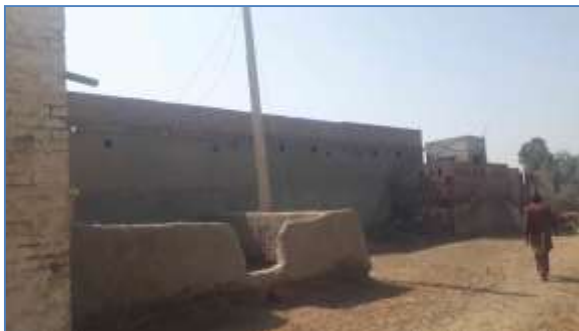
Plate 16: A view of affected structure at Nabi Bux , Tehsil Kandhkot and District Kashmore
