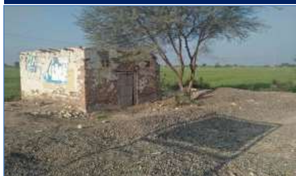
Plate 46: A view of right side affected structure at Goth Din Muhammad Mazari.
