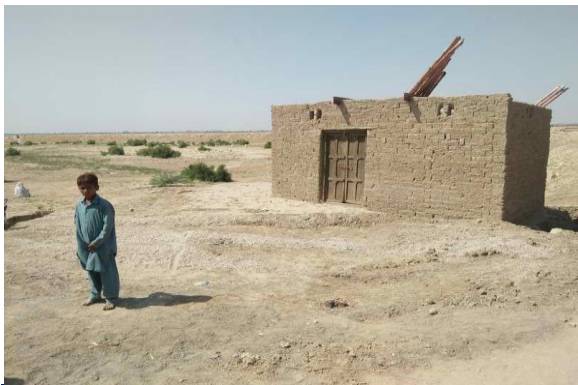
Plate 39: A view of affected structure located within the road RoW at Shah wali, Tehsil Rojhan, and District Rajanpur
