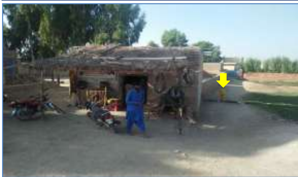
Plate 27: A view of affected structure left side and installing ROW markers project road section at Goth Qadir Bux, Shikarpur
