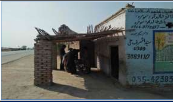
Plate 48: A view of affected structure at Machi Bindo, UC Jamal, Shikarpur
