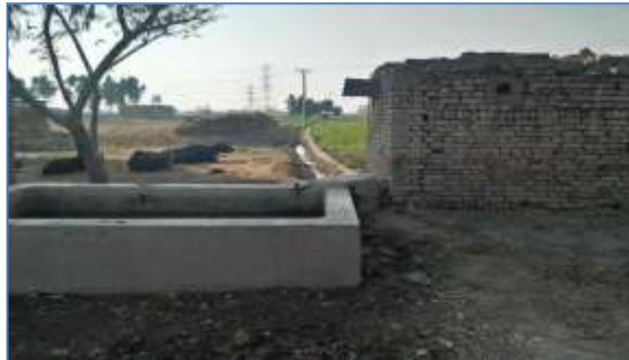
Plate 38: A view of affected tubewell
