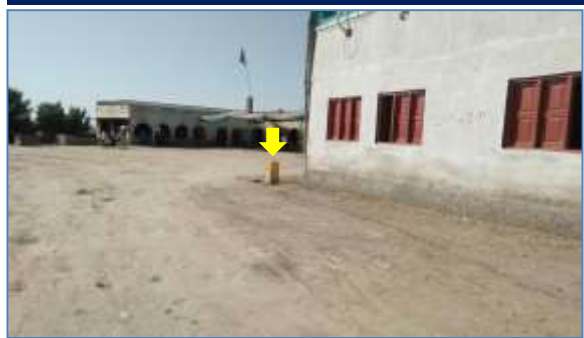
Plate 30: A view of installing ROW markers project road section at Chaninage 74+810 Karampur Laro
